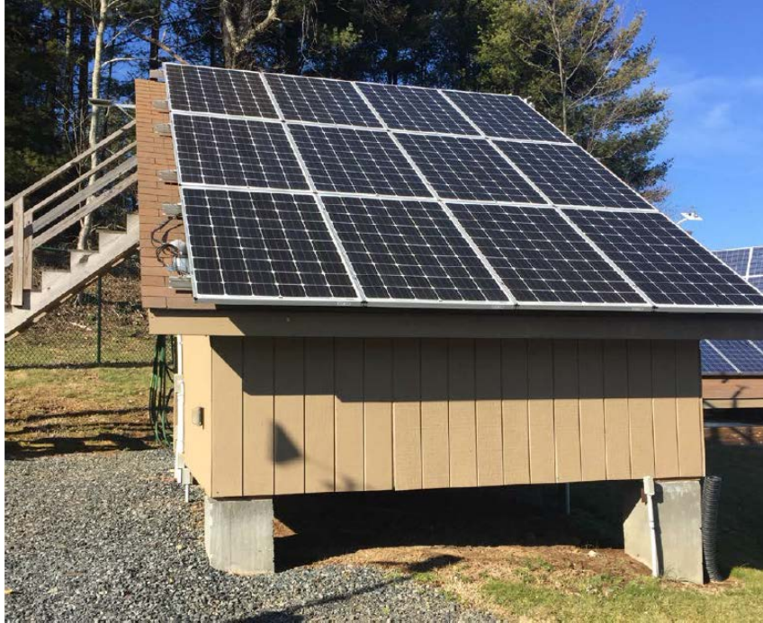
Figure 12. 3.36 kW PV array, Appalachian State Solar Lab.
