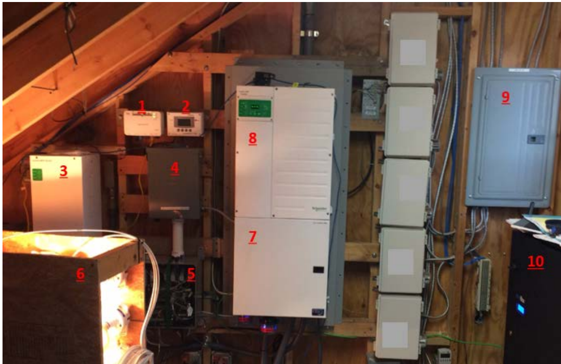
Figure 13. Self-Consumption system components, Appalachian State Solar Lab.
